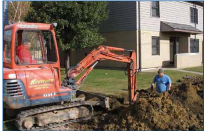
A backhoe is shown digging the trench for the new underground power lines at the John E. Horan Garden Apartments. The new lines replace the 70-year-old overhead lines that were often knocked out of service by high winds and ice storms.
